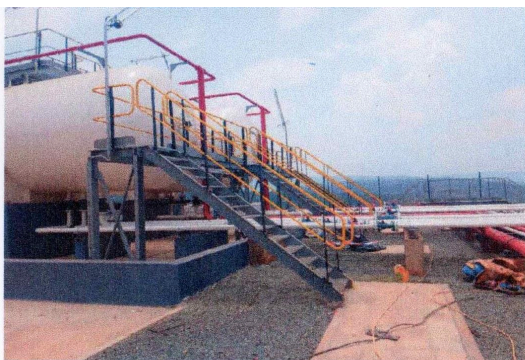
Handrails, staircases and LPG bullet gantries
