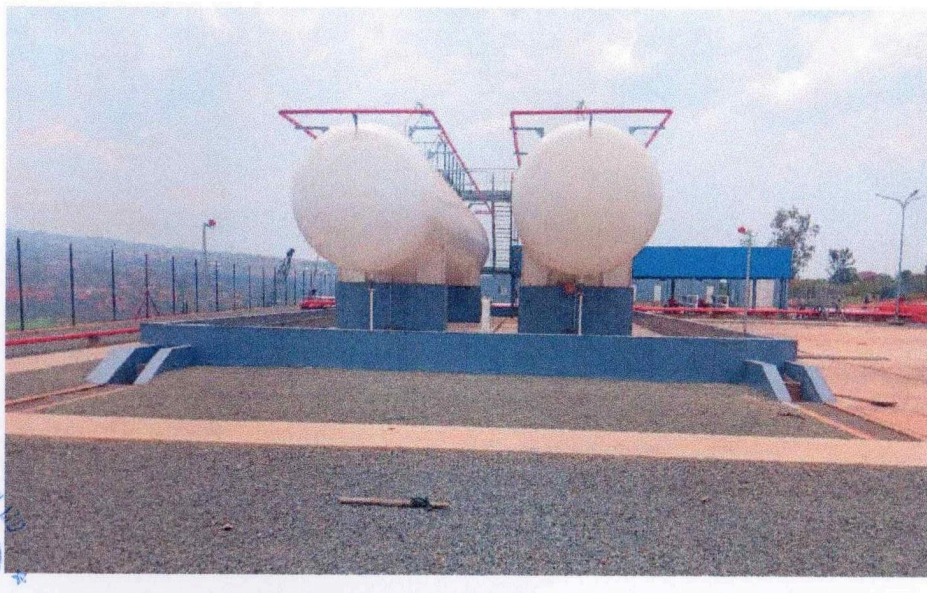
LPG storage spheres and bunded compound — 17,100 m 3 LPG storage & distribution plant, Rusororo
