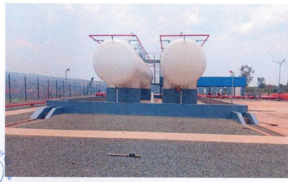
Completed LPG storage spheres and bunded compound
